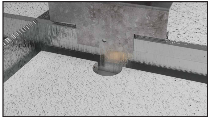
2 Create a notch in the ceiling tile for 1/2" conduit to pass through.
