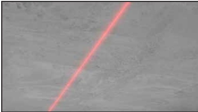
1 Scibe a line where the fixture will be place and make off hole locations according to shop drawing
